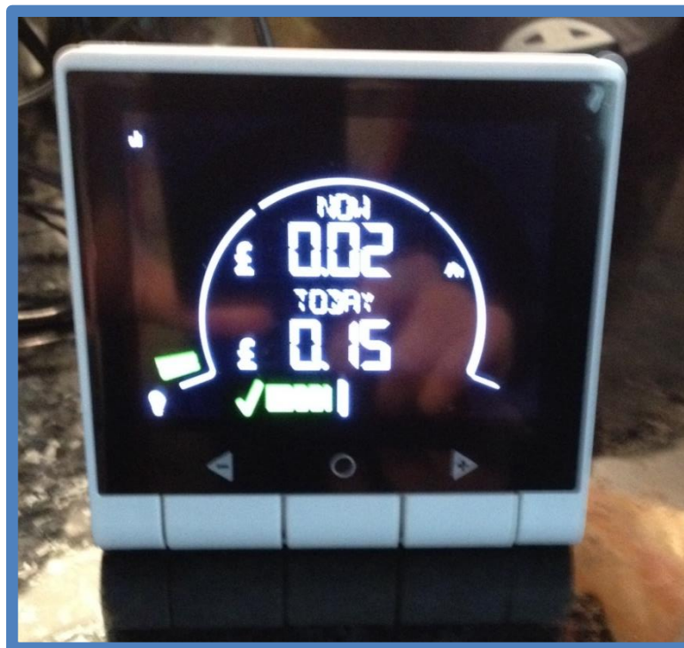
Figure 6: A plugged in, functional energy monitor
